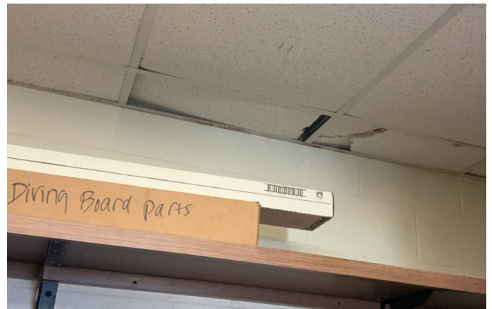
Independence Park East: Community Pool Storage Room
