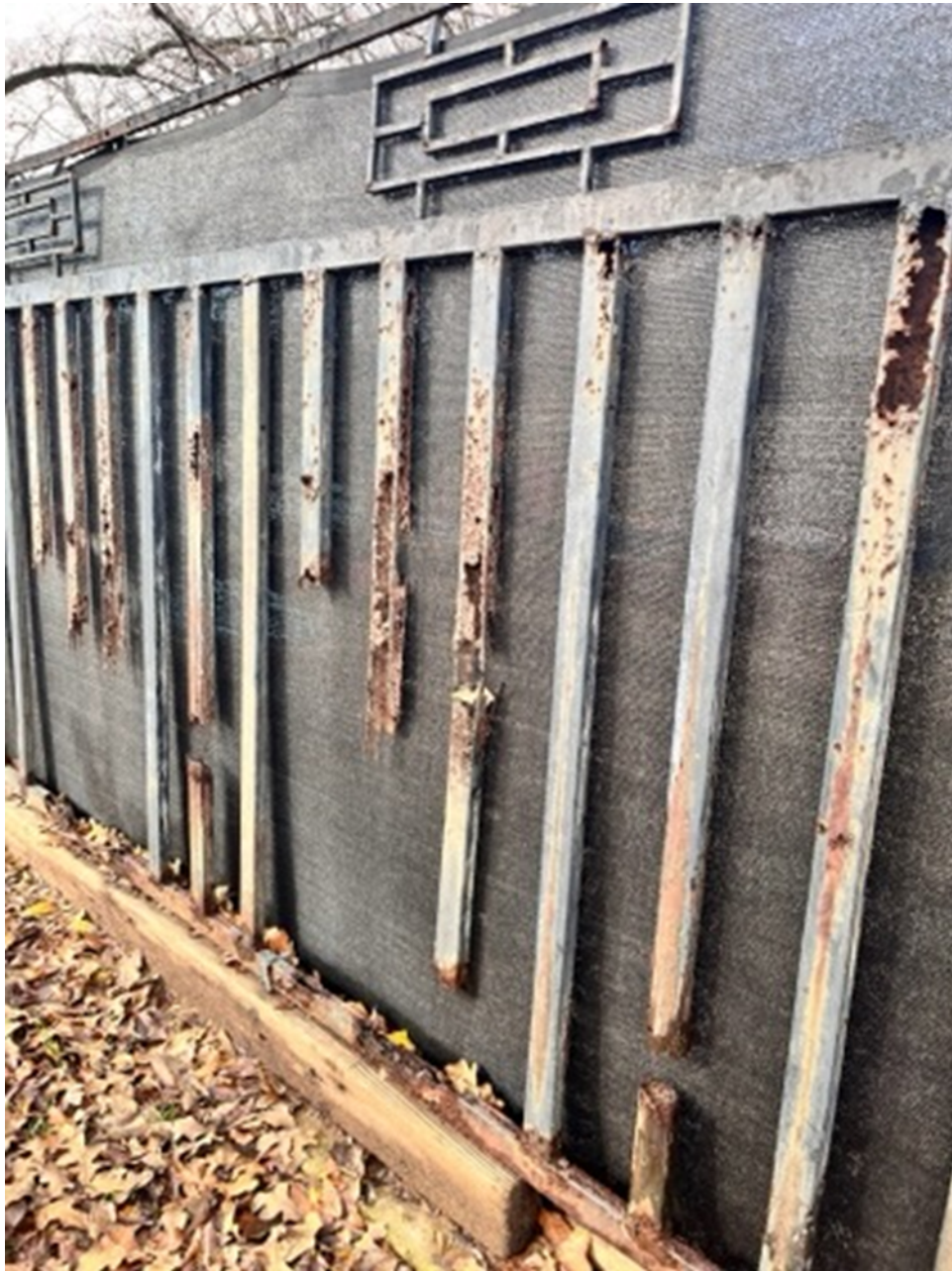
Exhibit D -Photos of existing deteriorating metal fence adjacent to rear property:
