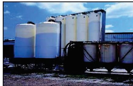
Large cone bottom tanks ranging in sizes from 2,500 to 13,000 gallons, are used to store and deliver up to 10,000 cubic ft. of bulk resins at a processing plant.
