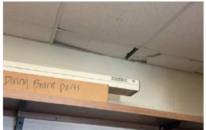
Independence Park East: Community Pool Storage Room
